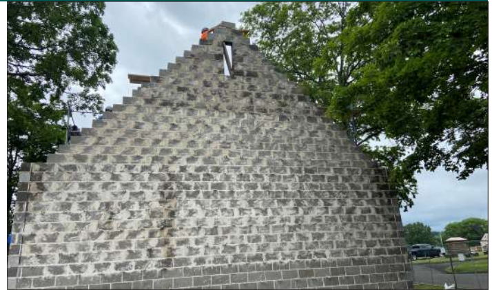
Munger Construction Company supervises placement of the last block on top of the Crematory extension wall.
